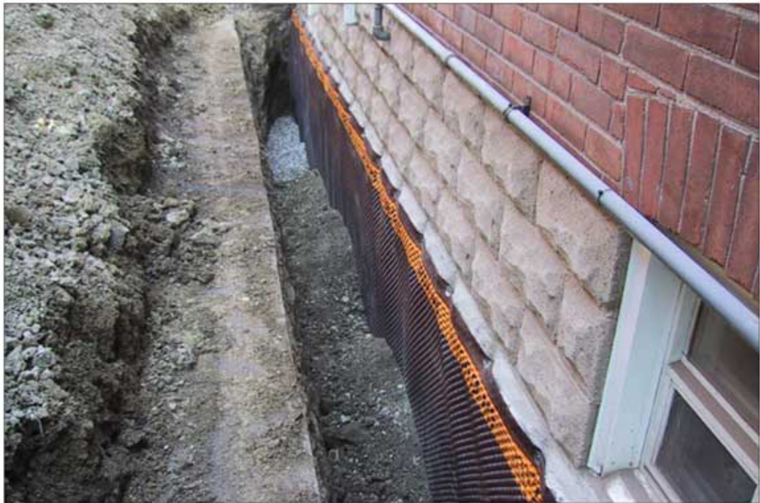
Part of the exterior waterproofing shows above ground. Houses are under constant hydrostatic pressure — which means water's always trying to get in.
